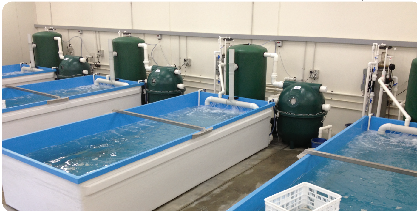
DF filters in an aquaculture facility
